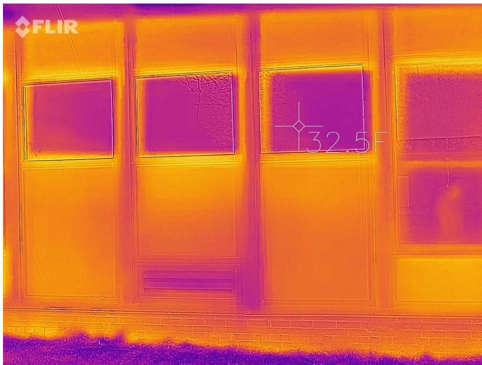
Figure 3: thermographic image indicating heat loss through panels is larger than through windows
