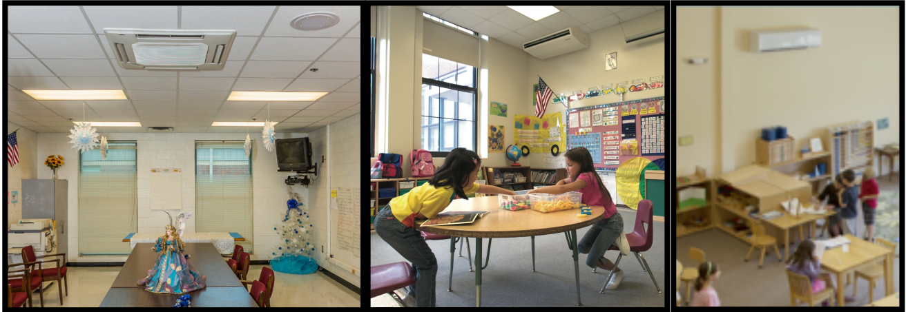
Figure 5: Indoor units in classroom settings: 4-way ceiling cassette, ceiling mounted unit, wall mounted unit
