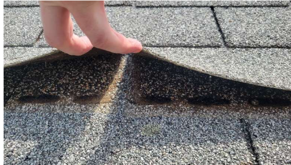
SEAL FAILURE COMMON
