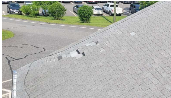
BROKEN AND MISSING SHINGLES
