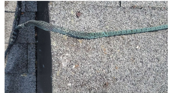
MISSING CAPS AND EXPOSED NAILS
