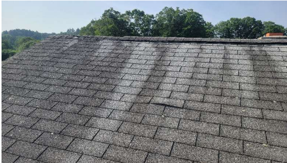
GRANULE LOSS AND DELAMINATION
