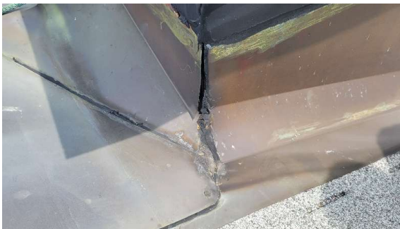
FAILED FLASHING SEAMS
