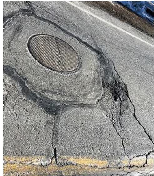
Figure 5. Freeze-thaw cycles lead to deteriorating road conditions. (Photo by Vicky Jenkins)
