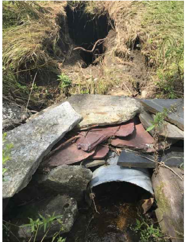
Figure 6. A culvert on West Gill Road in critical condition as of the 2023 FRCOG culvert survey. (FRCOG photo)
