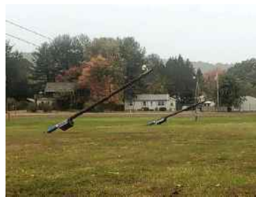
Damage from heavy winds & a thunderstorm at the Franklin County Fairgrounds, October 2020
